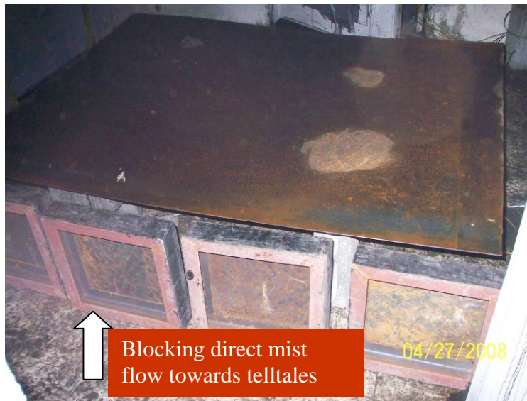
Figure 10: Direct flow of mist underneath the raised-floor was blocked
